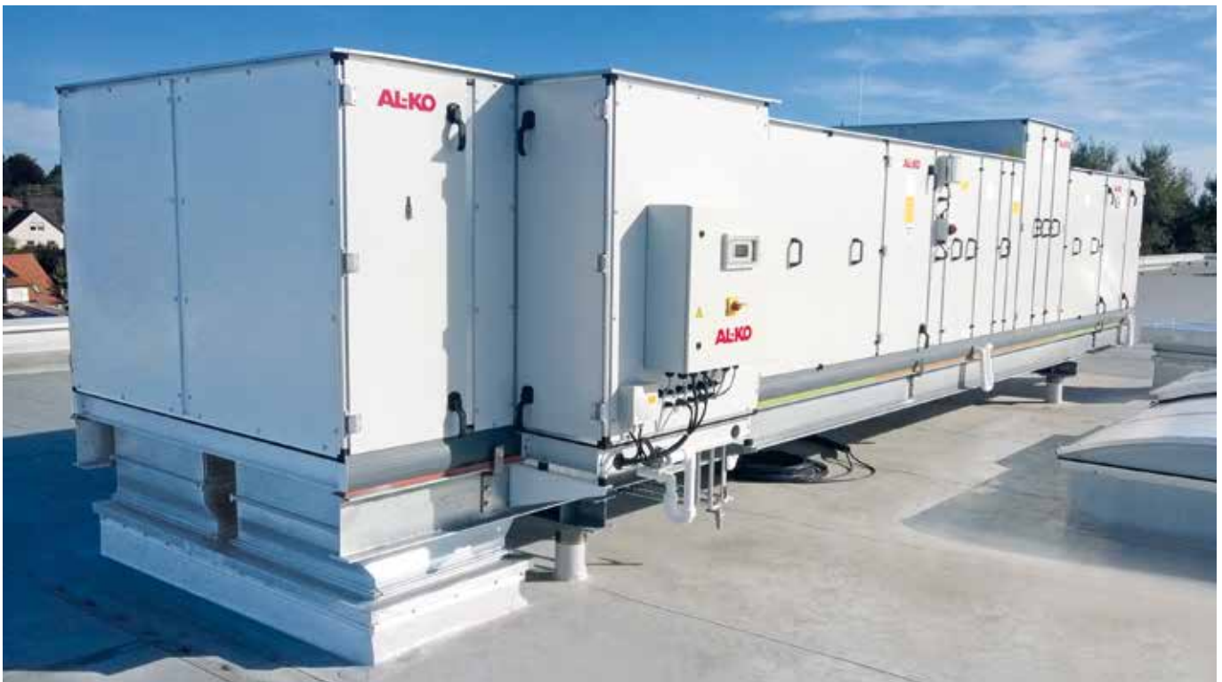
AL-KO Technology Centre in Kötz: HYGRO-OPT membrane humidifier in use since 2015
